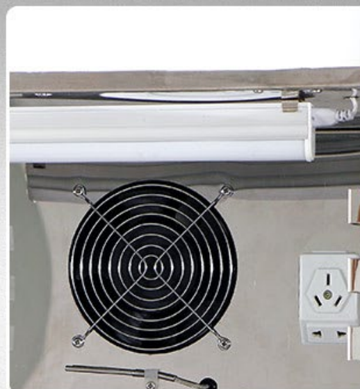
⊕ Lighting system and BOD socket
